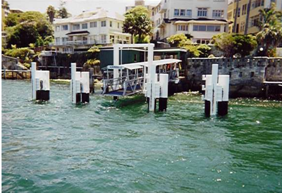
New Hydraulic Ferry Berthing Facility at Kirribilli Wharf State Transit Sydney Ferries
